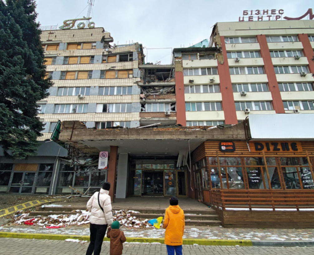
HOME AGAIN A woman and her children eye the damage to buildings near their apartment in Mykolaiv. They originally fled to Poland but returned this summer.
