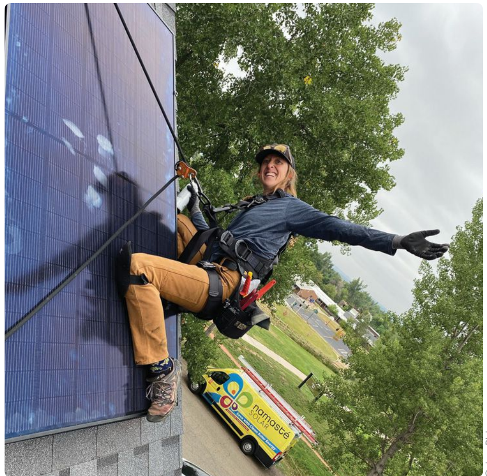
Riley Neugebauer, solar installer and apprentice at Namaste Solar, works on a residential solar project in Boulder, Colorado.
