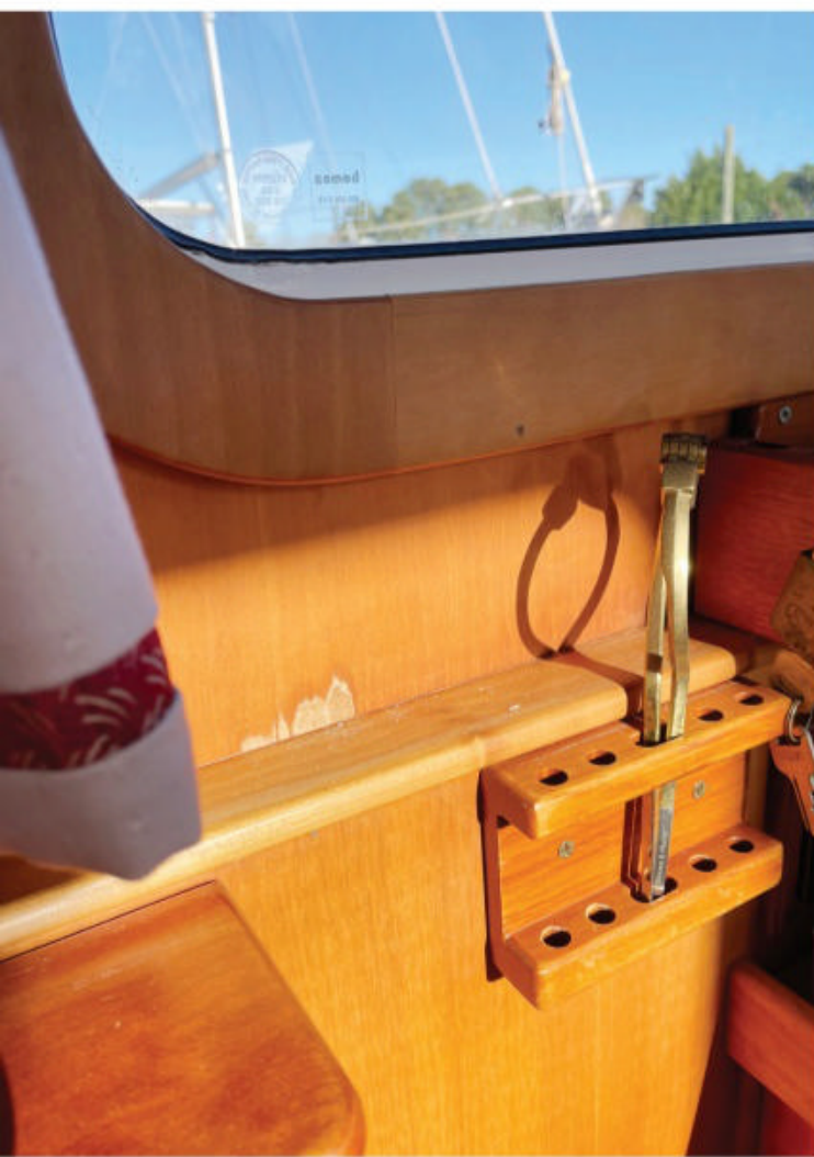
Discoloration beneath windows and ports is a sure sign it is time to remove and rebed them. A small freshwater leak can cause thousands of dollars of damage to interior veneers and substrates.
